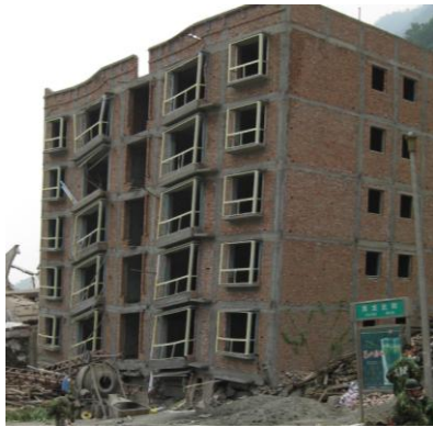
Fig. 11 First story of a constructing building collapsed
