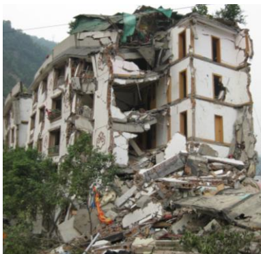
Fig. 4 Partly collapsed brick building
