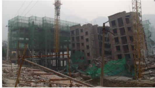
Fig. 12a Two constructing buildings, left, RC frame, some columns became hinge in 2 nd and 1 st stories, but still well stand there; right, BBF, 1 st story and central part collapsed
