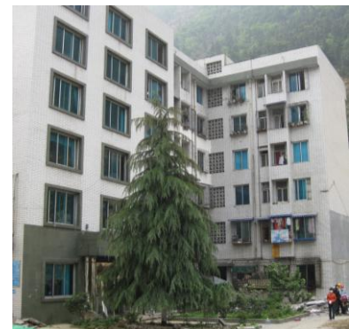
Fig. 6 Building keeps basic intact except one outwall hit by something
