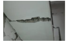
(b) Stairs almost break off
