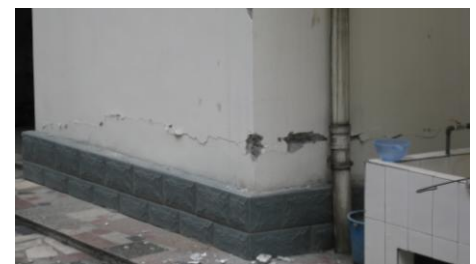
Fig.30 Horizontal crack of a brick building
