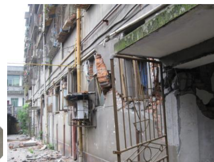
Fig. 38 first story of a six story BBF building heavy damaged
