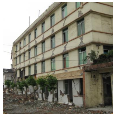
Fig.29 A brick building Heavy damaged at first story
