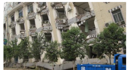
Fig. 9 First story of BBF building collapsed
