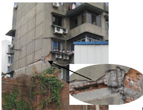
Fig. 37 Horizontal crack and dislocation at the bottom of 3 rd story of a six story brick building
