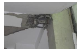
(c) Stairs beam end damage
