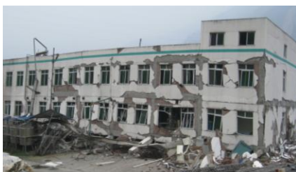
Fig. 16 First story of a three story frame workshop collapsed
