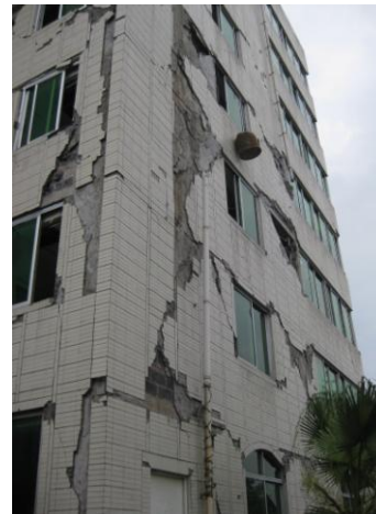
(a) Infill wall damage
