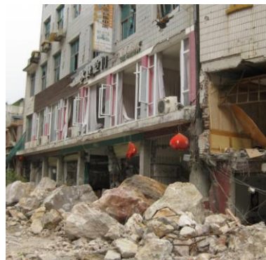
Fig. 5 Buildings damaged mainly by rolling stones, left-frame, right-BBF
