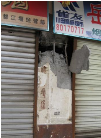
Fig. 31 Column damage of a BBF building
