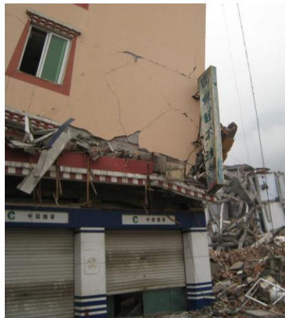
Fig. 14 2 nd story of a five story BBF building collapsed
