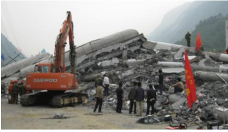
Fig. 10 Eight story frame building collapsed
