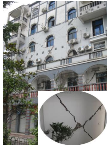
Fig. 32 Out and inner wall damages of a BBF building
