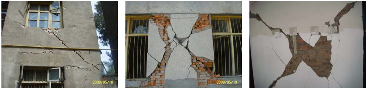
Figure 1 Typical phenomenon of through diagonal or X-shape cracks on the wall
