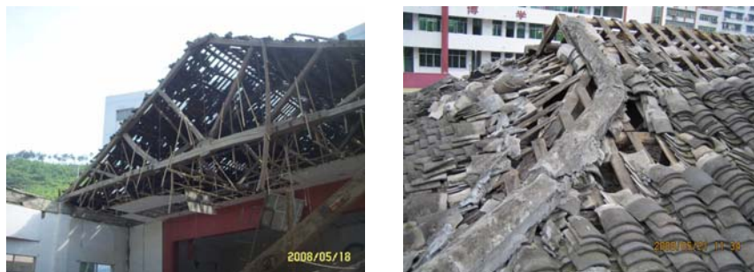
Figure 4 Damage of the wooden truss
