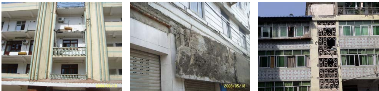
Figure 8 Typical damages of nonstructural components
