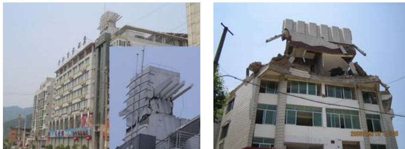
Figure 15 Severe damages of protruding members on the roof
