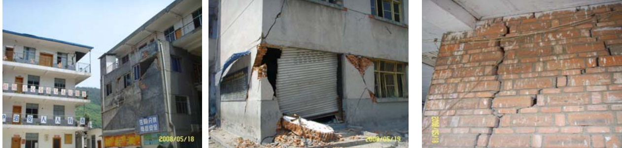
Figure 12 Partial damages caused by unauthorized reconstruction (closing balcony, demolishing and remodeling wall)
