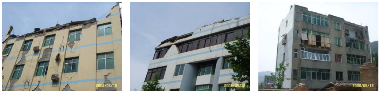
Figure 7 Partial collapse and fall of the parapet wall
