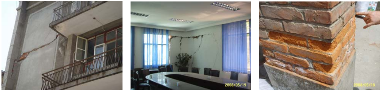
Figure 2 Horizontal cracks on the wall or the bearing brick column
