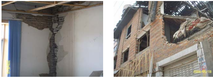
Figure 3 Separation of walls at the intersection of walls
