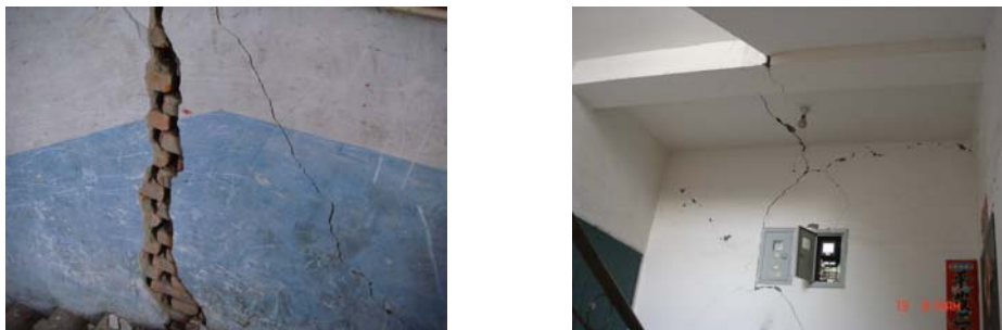
Figure 5 Typical damage of bearing wall and concrete slab in the stair part
