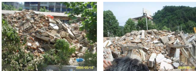
Figure 11 The wrecks of a collapsed 5 storey masonry building supported by reinforced concrete frame in bottom
