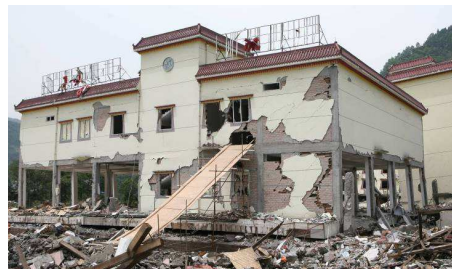
Figure 6 Partial collapse of 3-story RC frame building with masonry infill walls in Yingxiu
