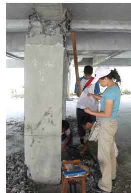
(c) Typical column damage
