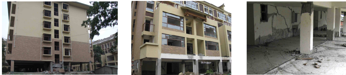
(a) Major damage (b) Moderate damage (c) Infill and column damages Figure 5 Variability of building response after Wenchuan earthquake
