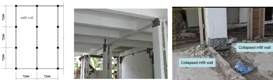
(a) Partial plan view (b) Column plastic hinging (c) Collapsed infill walls Figure 8 Views from a commercial RC frame building in Dujiangyan
