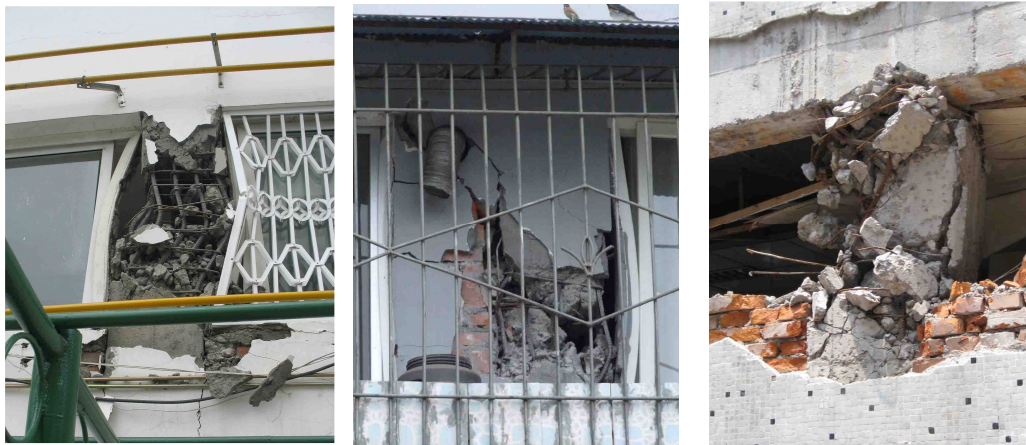
(a) Windows in both sides (b) Infill in one side only (c) Partial infills in both sides Figure 11 Short columns observed after the Wenchuan earthquake
