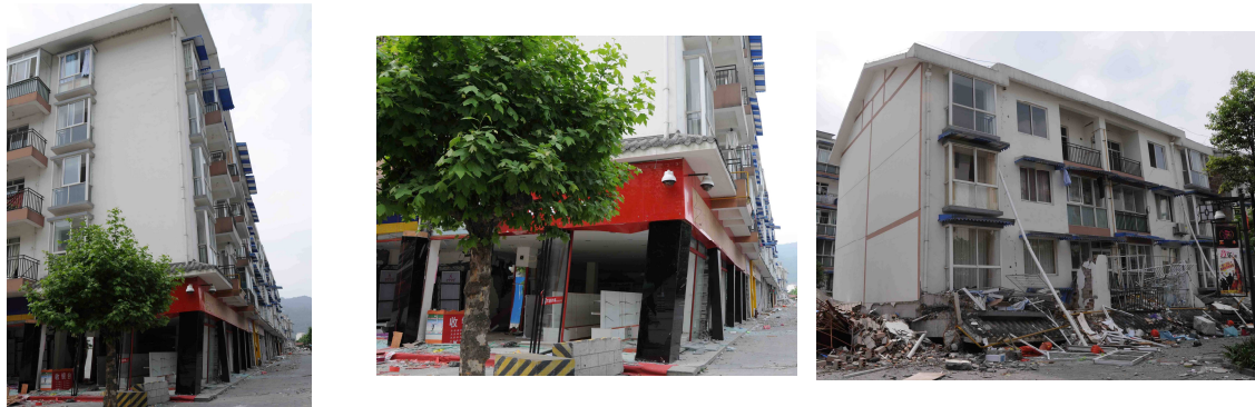
(a) Damaged 5-story building (b) Close-up of 1 st story damage (c) Collapsed 5-story building Figure 7 Views from two 5-story RC frame apartment buildings in Dujiangyan
