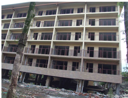
(a) Leaned 6-story building in Dujiangyan
