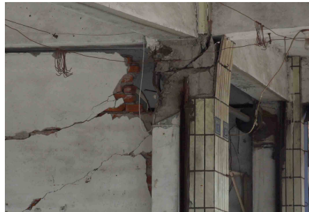
(a) Photograph of infill and column damages
