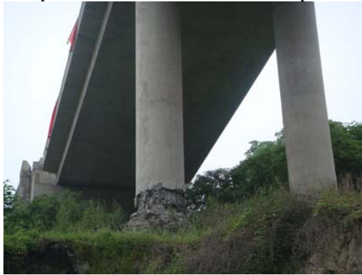
Fig.4 Rupture of concrete at Pier P1
