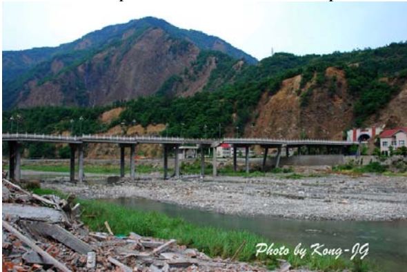
Fig.8 Shisuoyi Bridge deck moved severely
