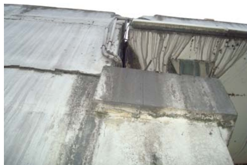
Fig.13 Crack on the wing wall of abutment
