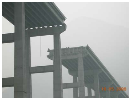
Fig.12 Left is 3# girder, right is 5# girder, 4# girder fell
