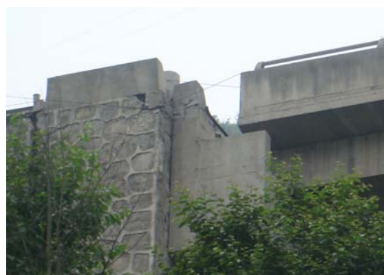
Fig.3 Crack on the wing wall of Abutment A1
