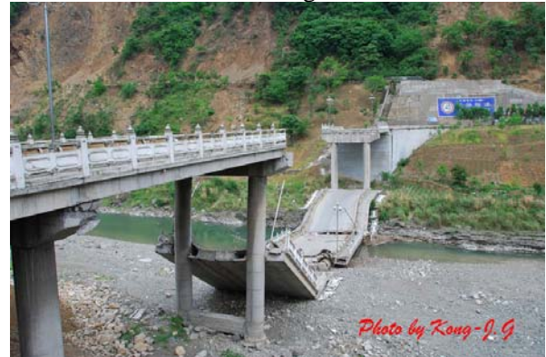
Fig.9 Fall of 3# -5#girder of Xiayu Bridge
