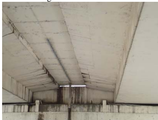
Fig.14 Damage of expansion joint
