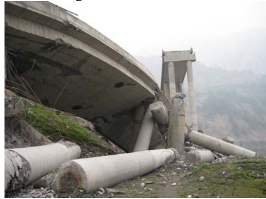
Fig.5 Fall of 2# girder
