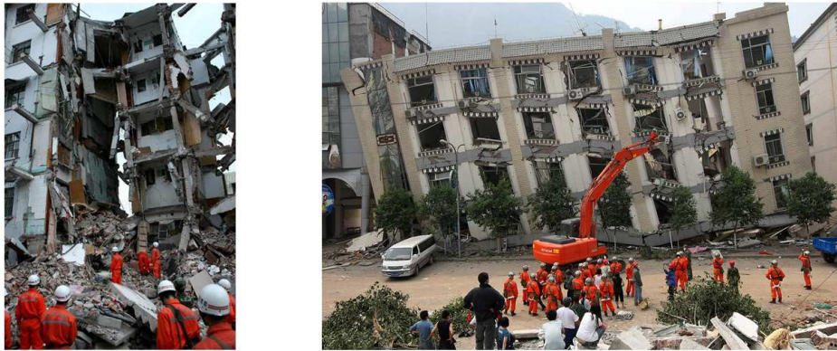
Figures 1 & 2 – Earthquake collapsed concrete buildings in Wenchuan, China, May 12, 2008 (Photos taken from http://xfj.zunyi.gov.cn/cms/cms/website )
