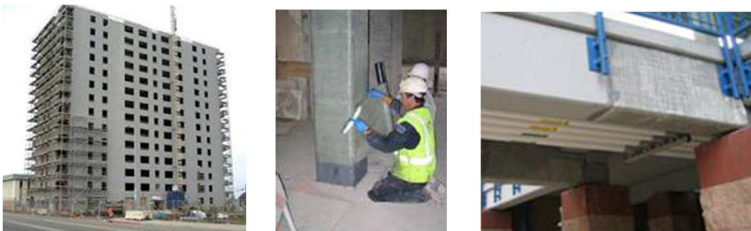
Figures 3, 4 & 5 – FRP seismic strengthening applications on walls, columns and beams (Courtesy photos from QuakeWrap, Tucson, AZ, USA)
