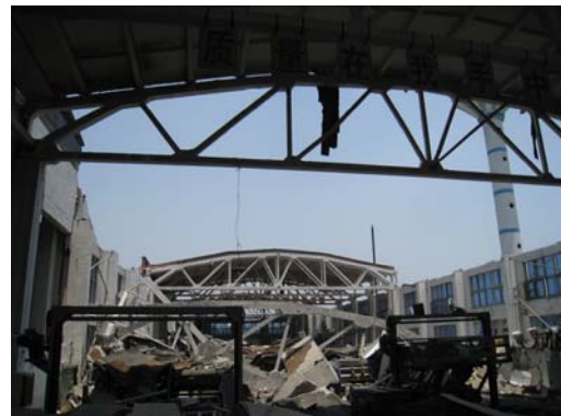
Figure 9 the local earthquake damage
