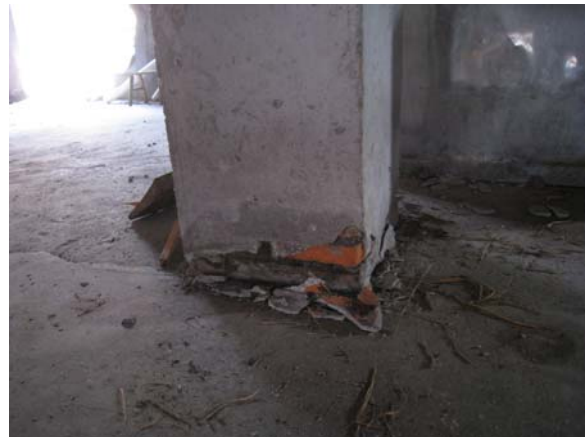
Figure 3 the local earthquake damage
