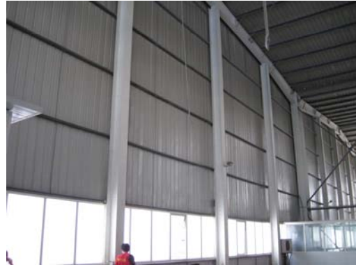
Figure 11 the local earthquake damage
