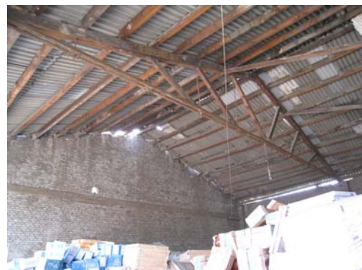
Figure 5 the local earthquake damage
