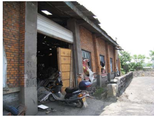
Figure 7 the local earthquake damage
