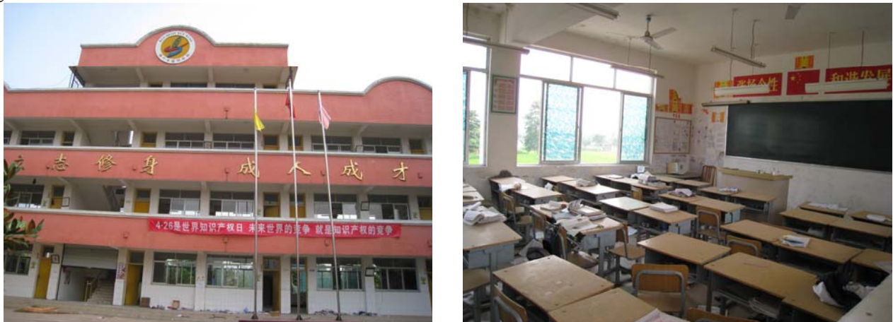
Figure 10 The major teaching building after the earthquake (outside and inside) (Photo by W. Wang)
