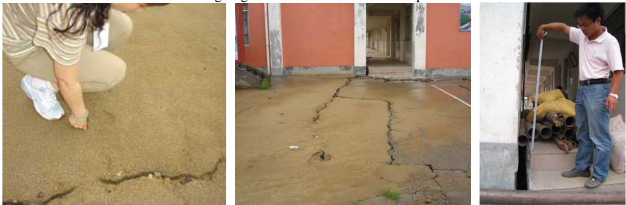
Figure 11 Sand boils and sandy soils ejected (Photo by Z. Cao)
