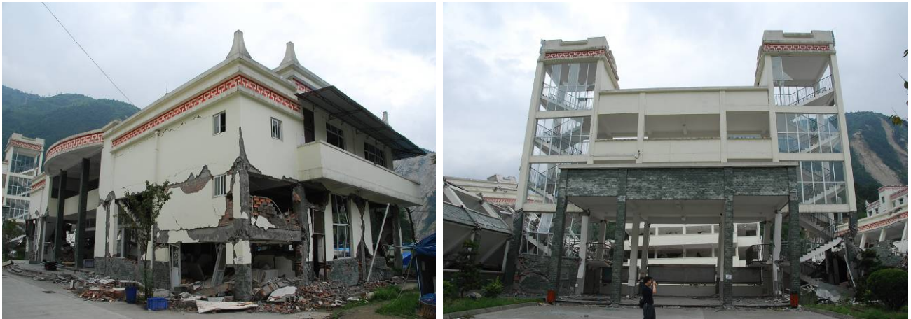
Fig.11 bottom story damage
