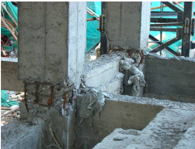
Fig.6b. beam-column damage of R/C frame
