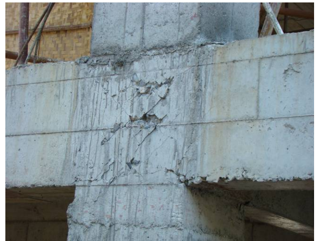
Fig.6c. beam-column damage of R/C frame
