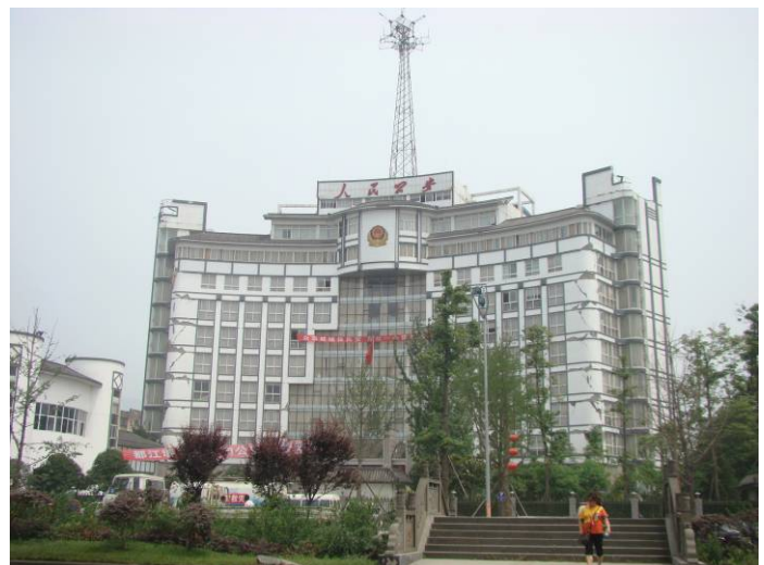
Fig.4 Building with serious damaged masonry infill
