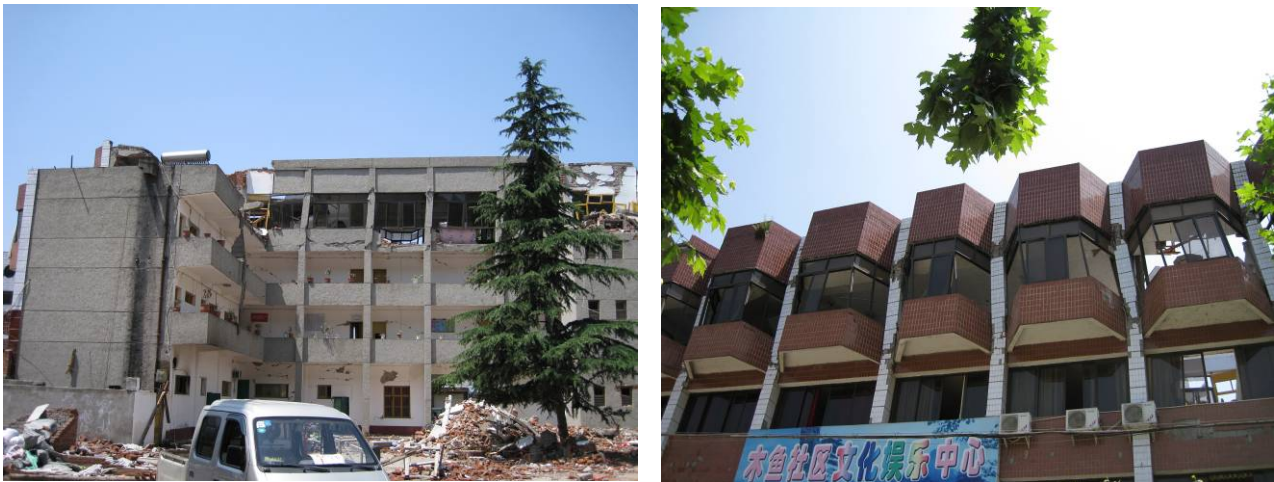
Fig.9 Top story damage
