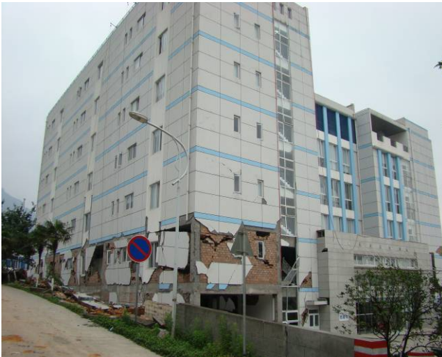
Fig.5 seriously damaged masonry infill
