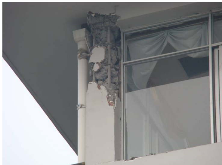
Fig.7 Column damage in top story
