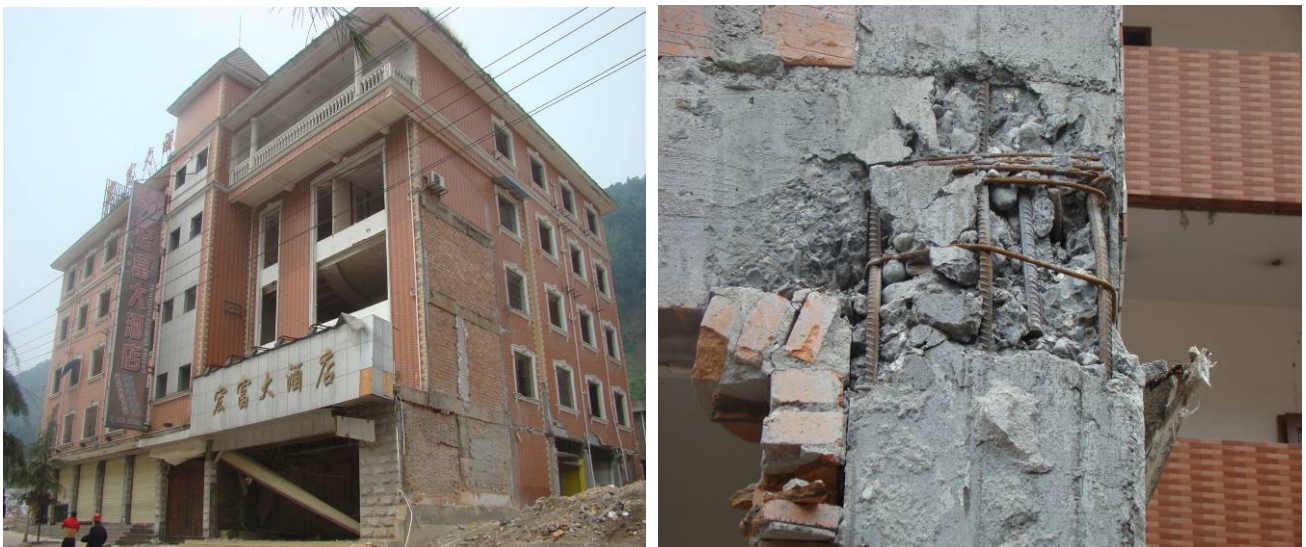
Fig.10 bottom story damage
