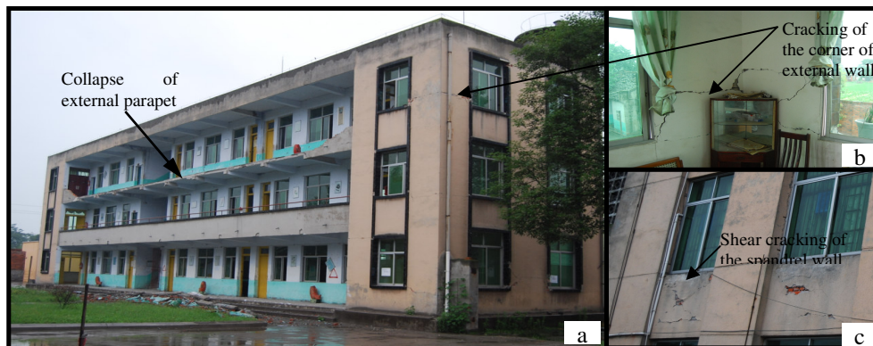
Figure 2 The damage of the main teaching building of the Centre Primary School of Mian yuan Town
