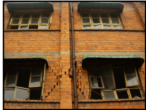
Figure 4 The collapse of the external wall
