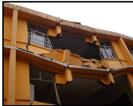
Figure 3 The collapse of the external wall of the teaching building of Hanwang Town Secondary School
